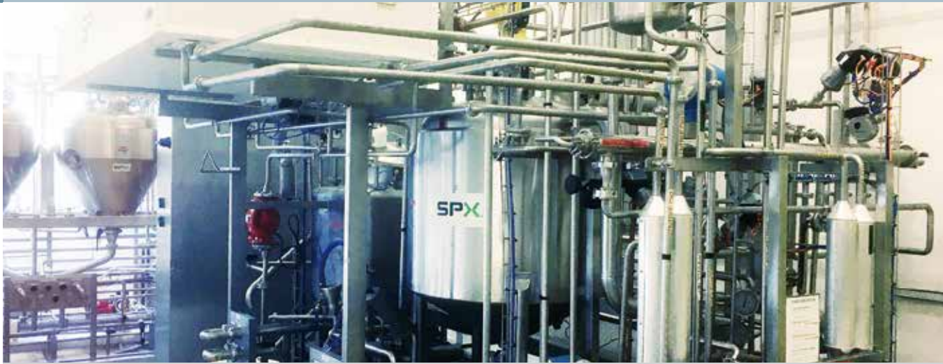
Fresh Dairy Pilot Plant, SPX FLOW Innovation Center, France
